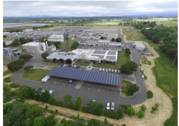
Figure 2. Laguna WWTP Carport Solar
