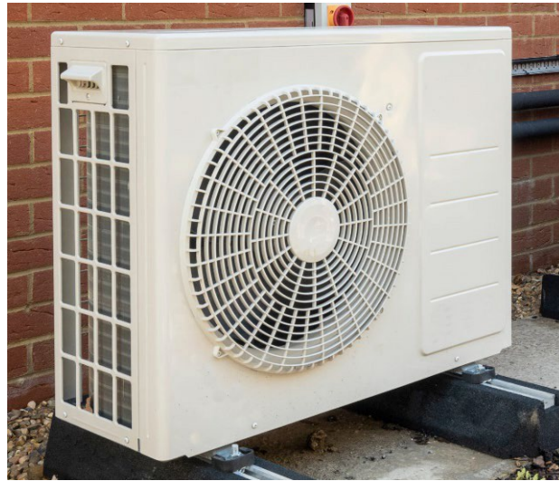
Heat Pump (exterior)
