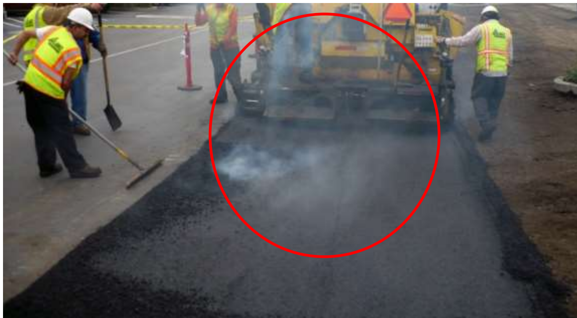
Figure D-1.3: Blue smoke from freshly laid pavement
