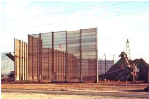
Figure IV-1: Typical Wind Screen - constructed to protect a down-wind stockpile.
