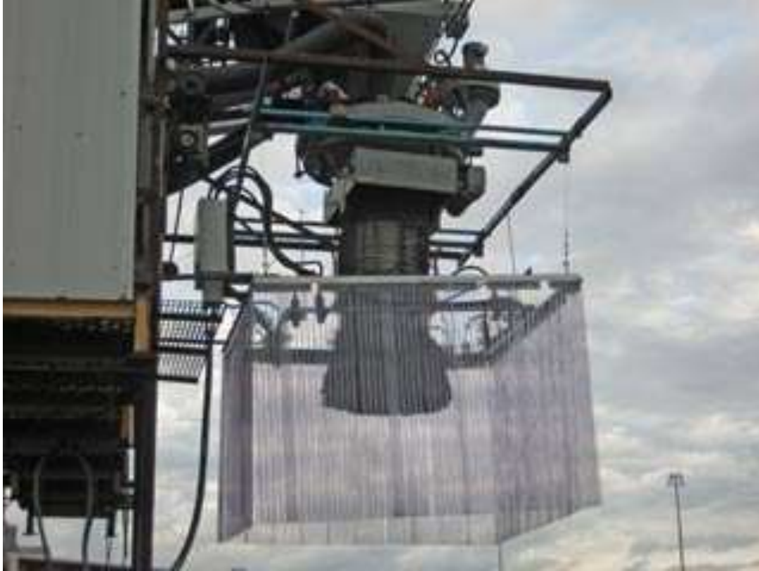
Figure IV-3: Wind Barrier surrounding a conveyor transfer point
