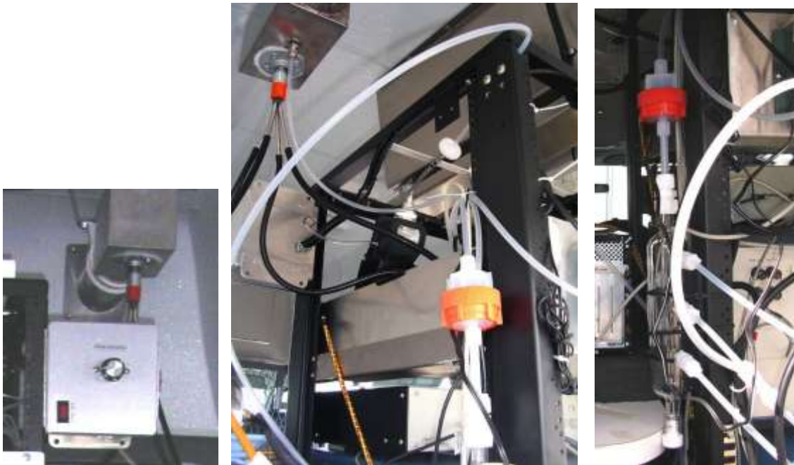
Photos of the inlet duct and fan control, stainless steel plenum exiting duct, and glass plenum with particle filter (replaceable paper disk filter is in the orange cartridge).
