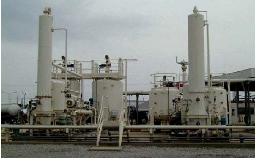
Figure 3 Example of Terminal Vapor Processing Unit
