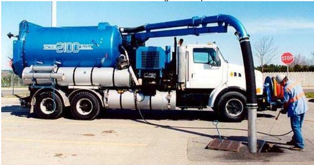
Figure 3 Vacuum Truck Servicing a Municipal Sewer
