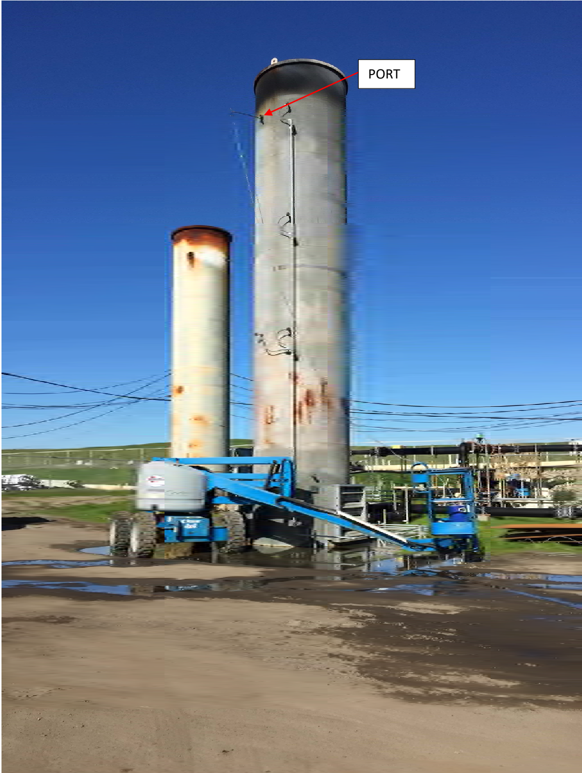
West Contra Costa Sanitary Landfill – Flare A161
