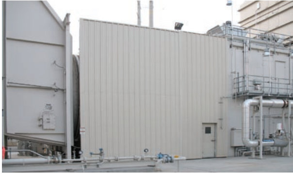
3. Sound-absorbing walls reduce noise generated by the gas turbines (left)
