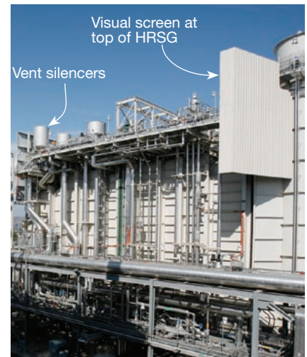
5. Vent silencers are of a squat design to restrict their height to 1 ft above the visual screen
