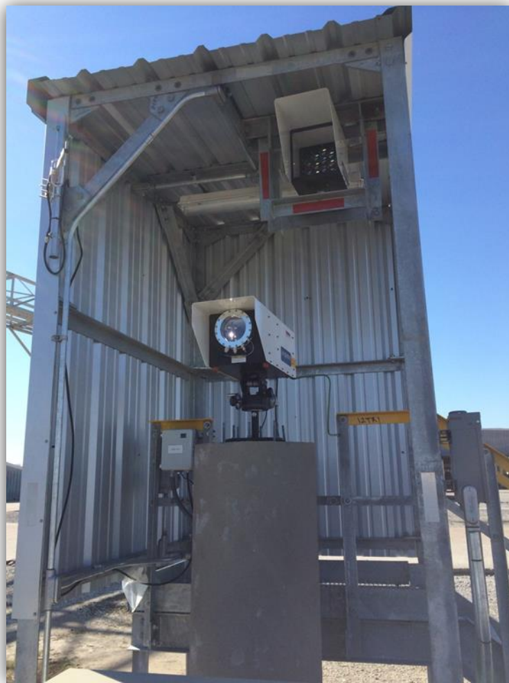
Figure 17. Example of a UV-DOAS analyzer installation.
