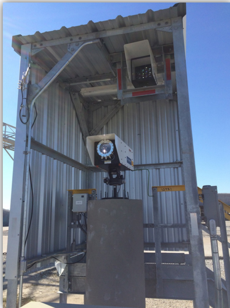
Figure 17. Example of a UV-DOAS analyzer installation.
