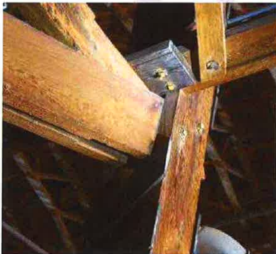
Figure 8. Example location of end split in cross brace member within Hangar 2.
