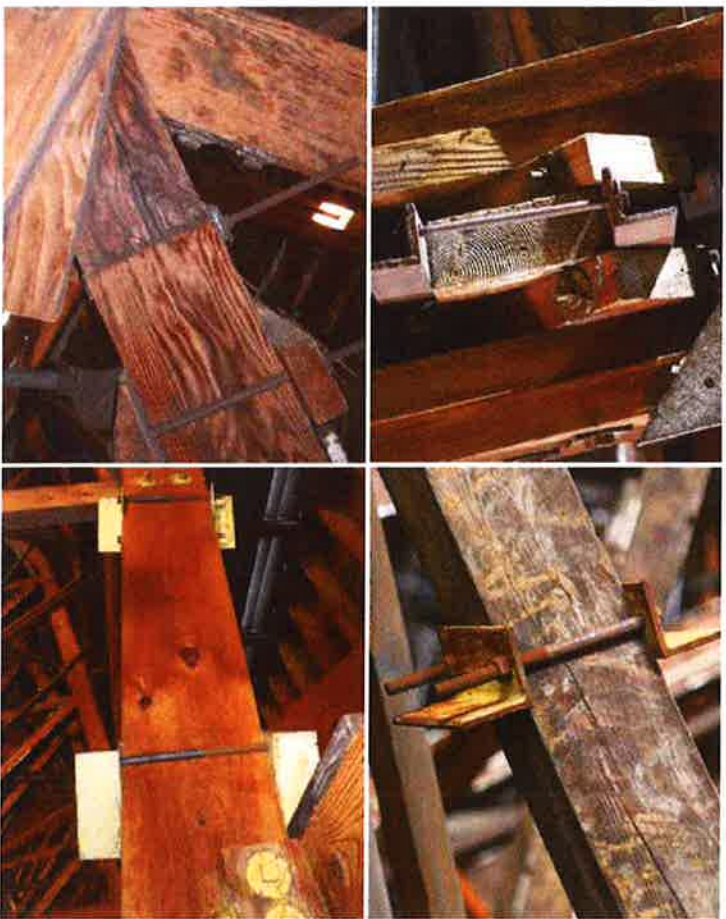
Minor repairs made during Hangar 3 service life
