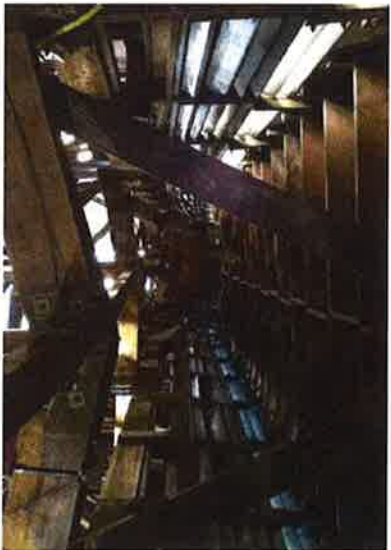
Roof monitor deflection in critical zone
