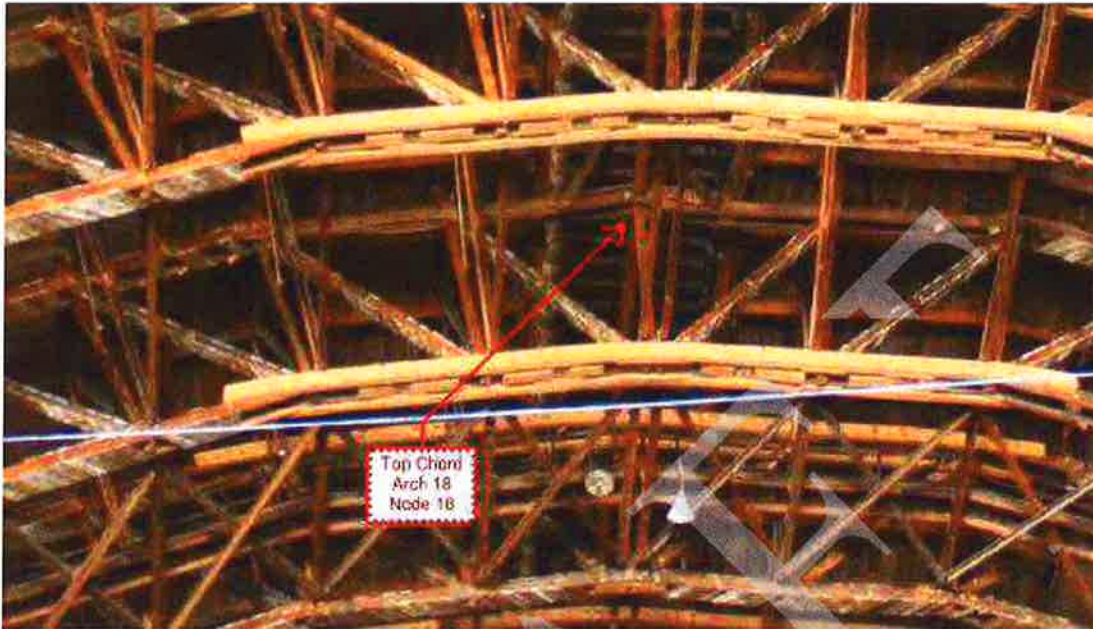
Figure 6. Observed cracks and lateral displacement of arch top chord in Hangar 3.
