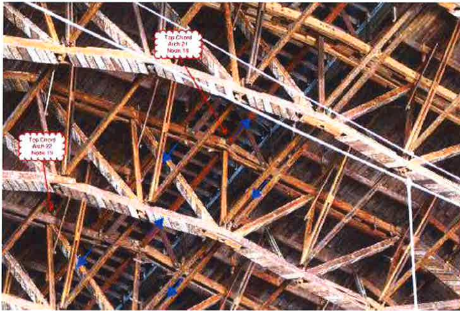
Figure 7. General trend of relative lateral displacement at the arch apex top chord in Hangar 3.
