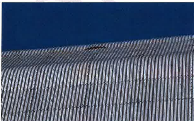
Figure 10. Example location of detached corrugated aluminum sheathing on roof exterior of Hangar 2.
