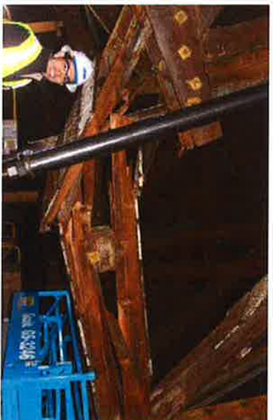
Damaged chord member viewed from access tower
