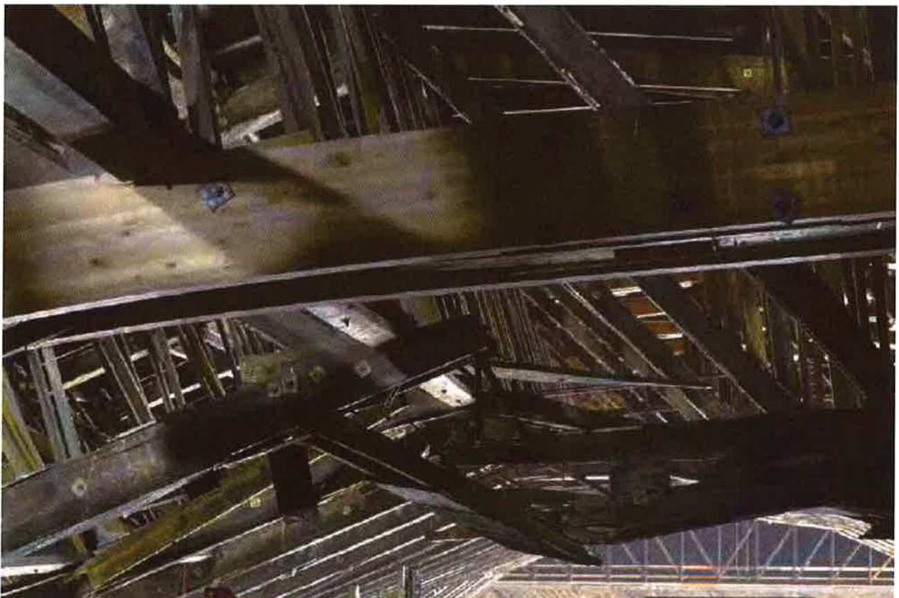
Figure 6. Broken bottom chord near top of truss.
