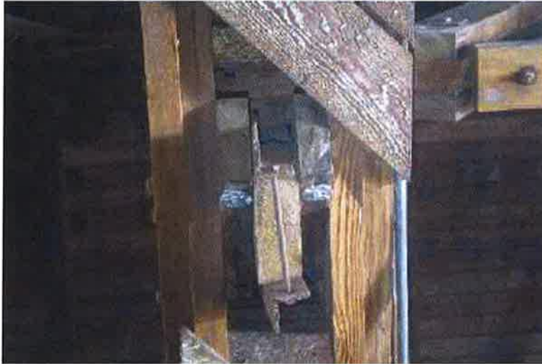
Figure 17. Example of new minor connection strengthening stitch bolts adjacent to existing angle clamp.
