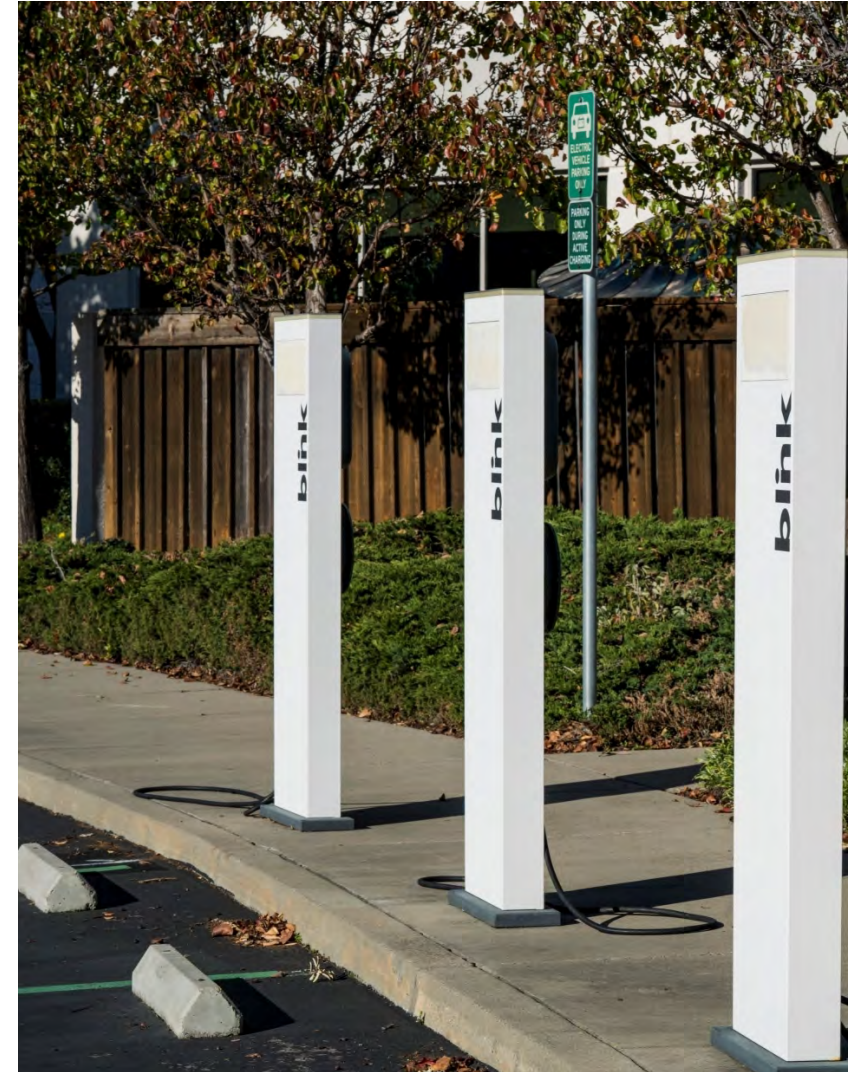
Electric vehicle charging stations. Bay Area Air Quality Management District.
