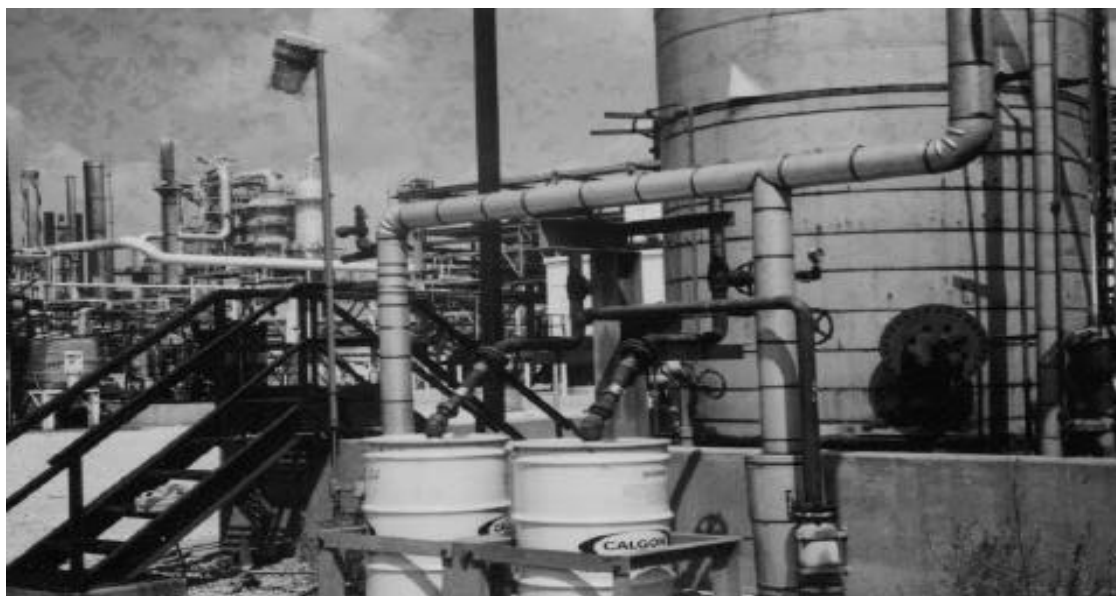
Figure 4 Use of Carbon Adsorption for Control of Wastewater Collection Systems at a Refinery 10
