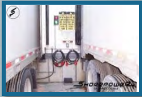
Loading Dock Power Plugs
