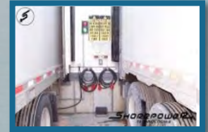
Loading Dock Power Plugs
