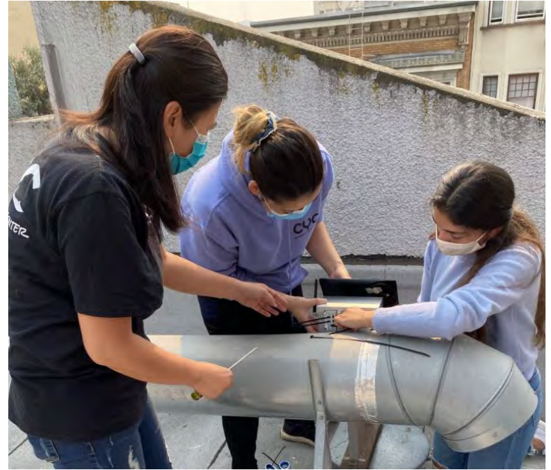
October 2020 - Sensor Installation at CYC Main Office
