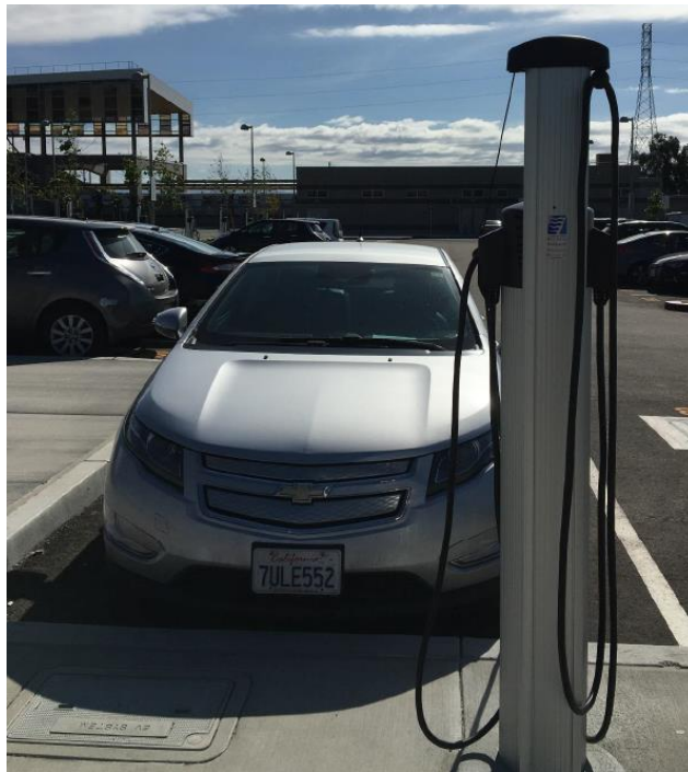
Figure 11. EV Charging Station at the Warm Springs BART Station
