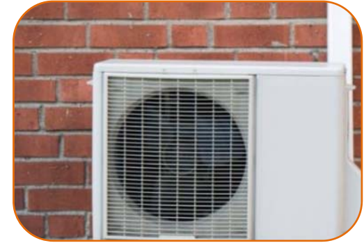
$3,500 electric heat pump
