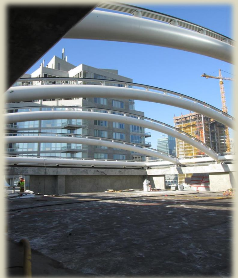
Figure 4: Atrium Skylight Support
