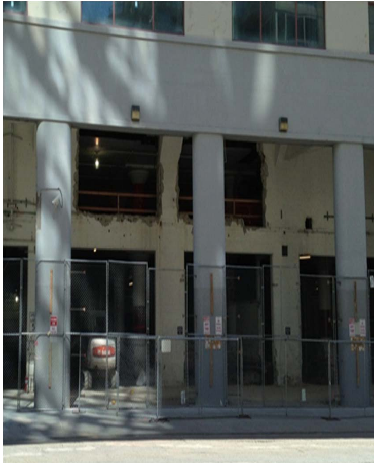
Beale Street entry: current condition.
