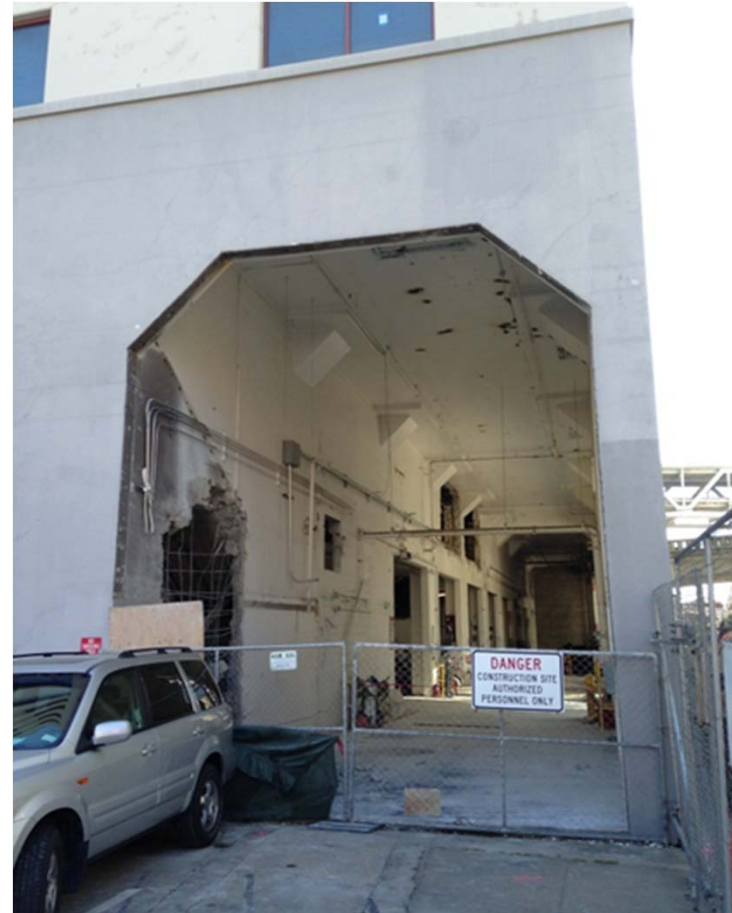
Corner of Rincon Place and Beale Street: this former railcar entry will be the future retail entry.
