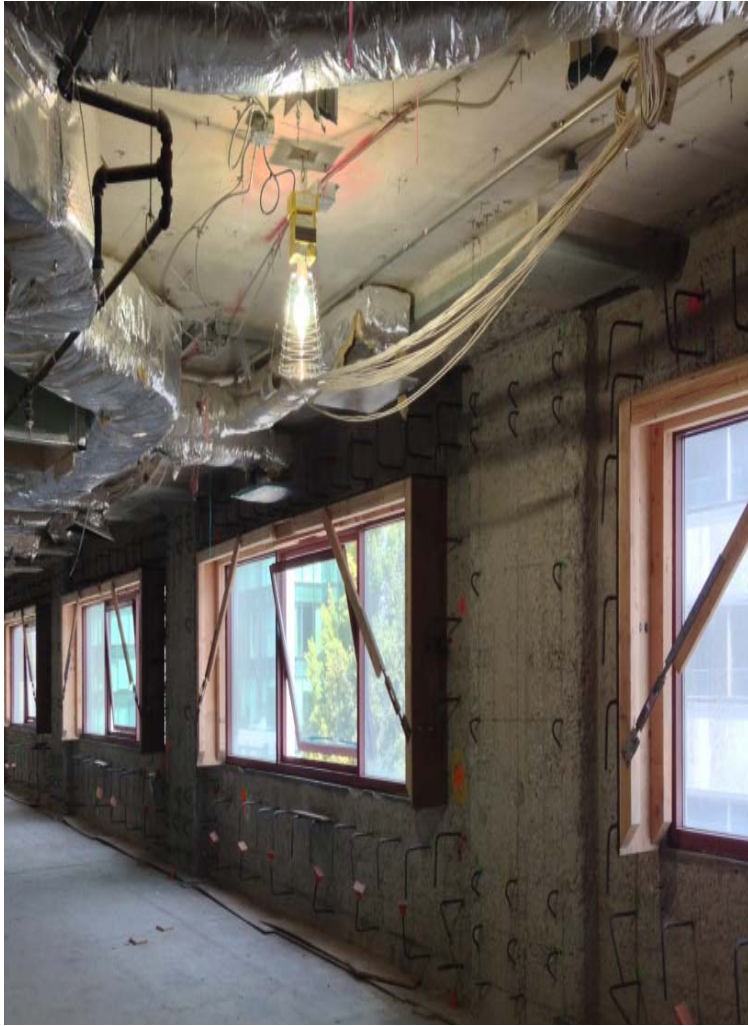
Rebar dowels installed on the perimeter walls. Concrete will be shot against the walls to seismically strengthen the building.
