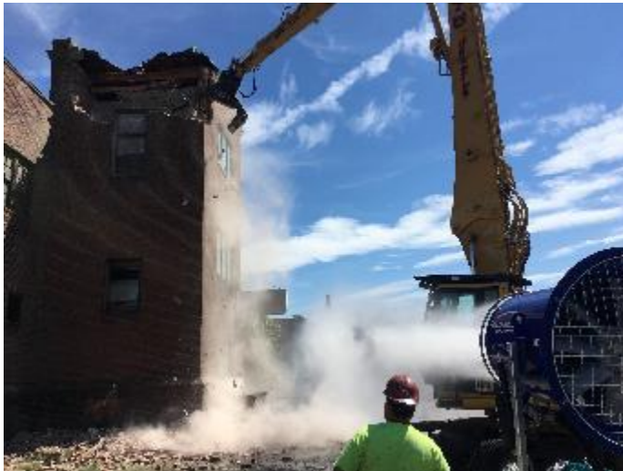
Construction and demolition can be a major source of particulate matter emissions
