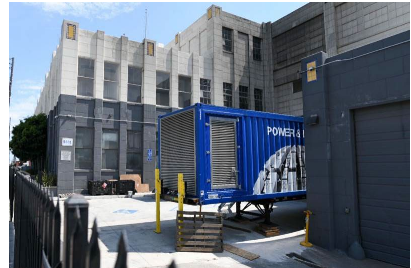
Figure 7: Unpermitted diesel-fueled generators supply power to now closed cannabis production facilities in East Oakland on July 28, 2022. (Source: https://www.kqed.org/news/11958266/after-lawsuit-managers-of-defunct-oakl Beth LaBerge/KQED)
