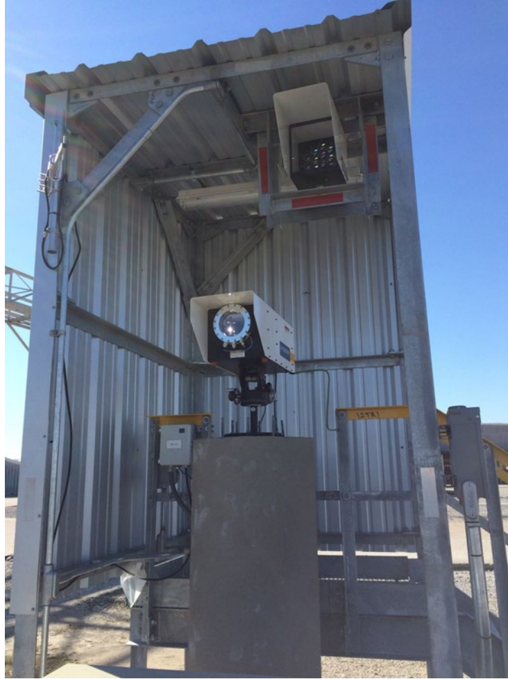
Figure 11. Example of a UV-DOAS analyzer installation.
